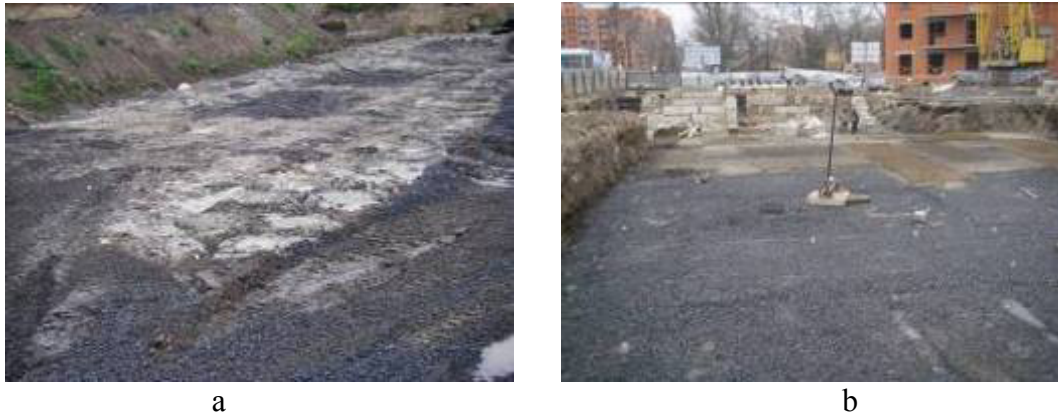
Figure 1 – The bottom of the foundation pit (sections IV and V) after reinforcing the SCE of the base (a), the gravel pillow, sprinkled on top of this base, and the strip monolithic foundations (b)
